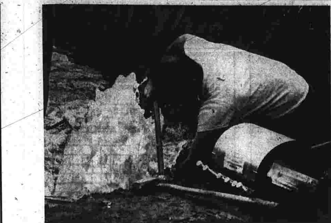
Henry Lester, a water department worker, clears an area around a leaking pipe so that a clamping sleeve can be slipped on to seal the break. (Herald photo by O'Hara).
